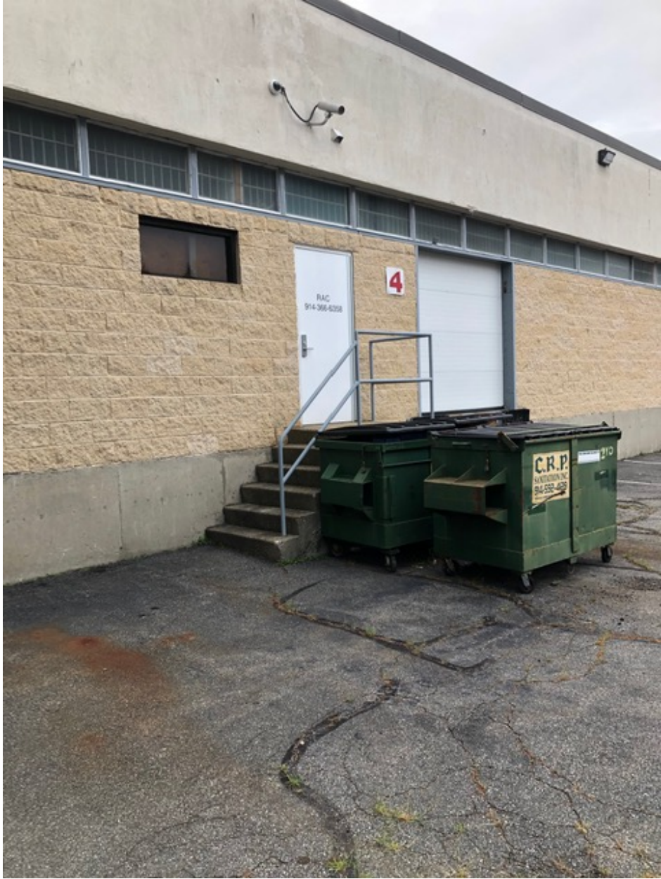
Photo 3: Affected area (note stair orientation)
