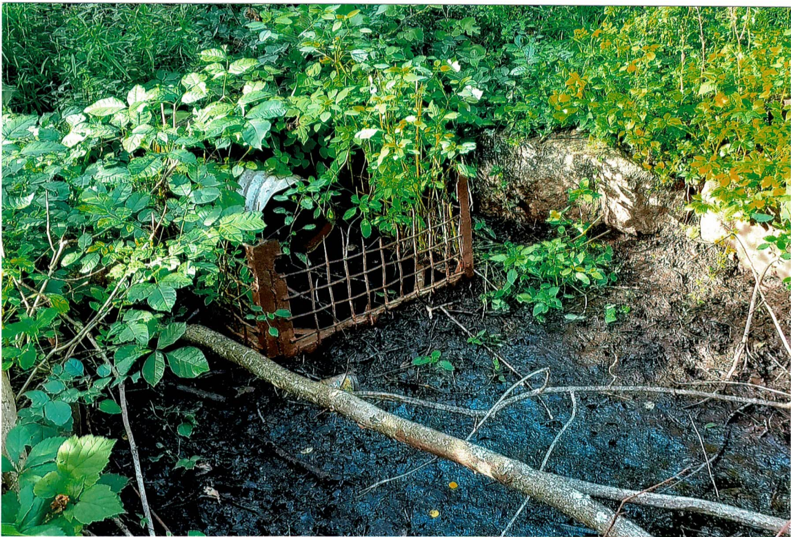
Photo 10 Looking toward drainage pipe with cage exposed at northern end of pond. Aug. 2021- The Cohen Site, 9 Hobby Farm Drive, North Castle, NY
