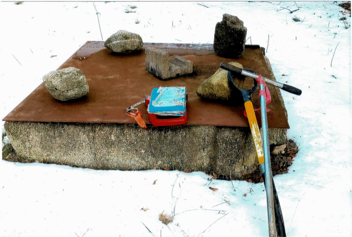
Photo 2 Looking toward fieldstone and concrete vault with metal cover located on the southwest corner of the site. Jan. 2022- The Melamed Architects Site, Byram Ridge Road, North Castle, NY
