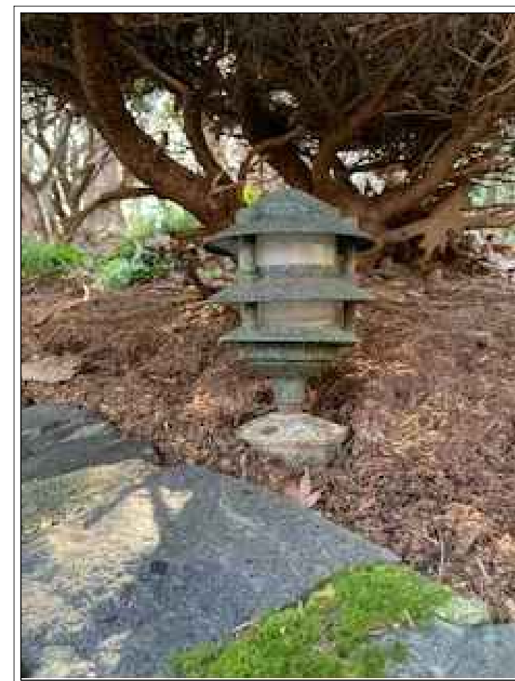
EXISTING PATH LIGHTS EXISTING PATH LIGHTS ARE USED FROM DUSK UNTIL APPROXIMATELY 9:00 PM.
