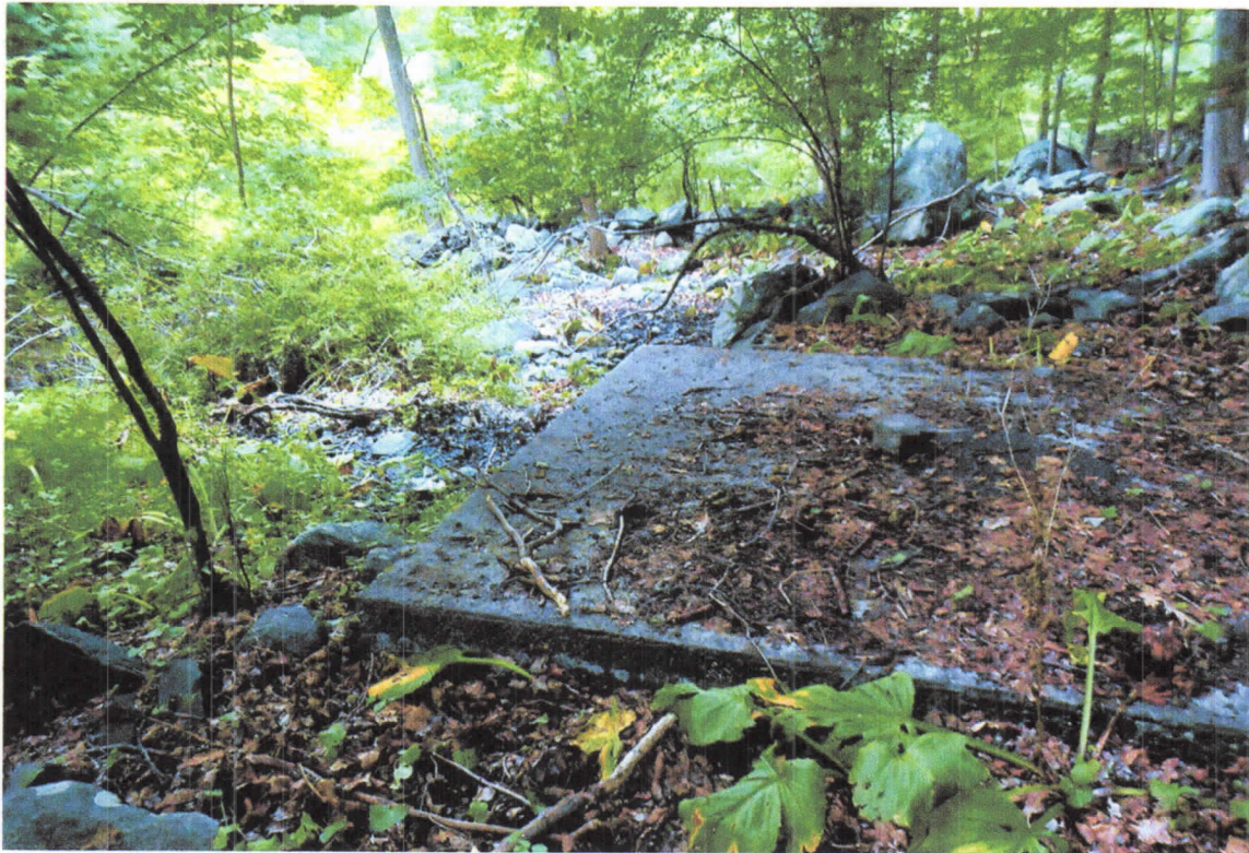
Photo 9 Looking southwest toward remains of pump / well house constructed of concrete and located on the southwest corner of the site.
