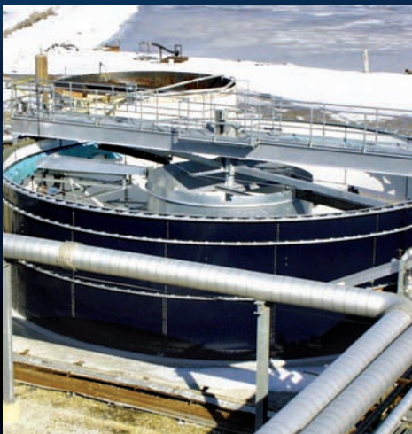
Wastewater Clarifier / Sludge / Storage / Mixing
