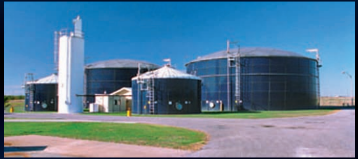
▲ Sludge stabilization and sludge storage facility.
