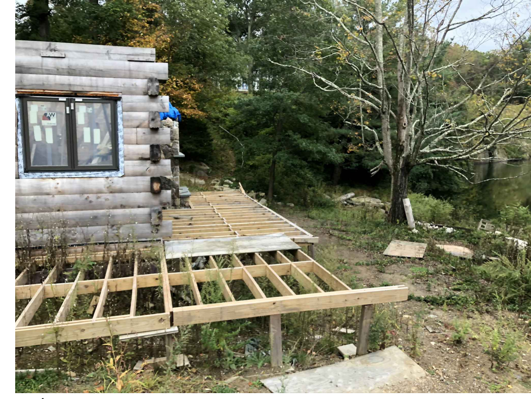
17 DAMAGED LAKESIDE CABIN REQUIRES RECONSTRUCTION. DILAPIDATED CABIN AND CABIN DECK HAVE BEEN REMOVED
