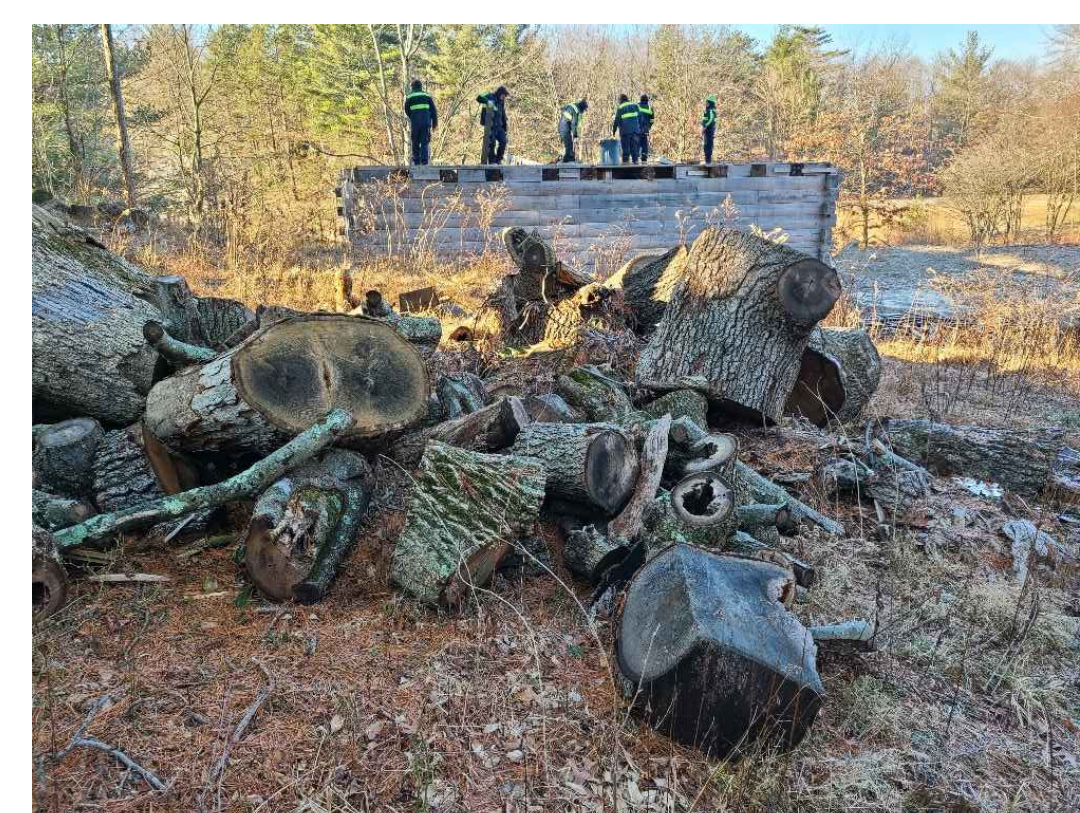
23 VIEW OF ADDITIONAL DEBRIS PILES NOW REMOVED. DAMAGED CABIN IN BACKGROUND HAS NOW BEEN REMOVED DOWN TO THE FOUNDATION.
