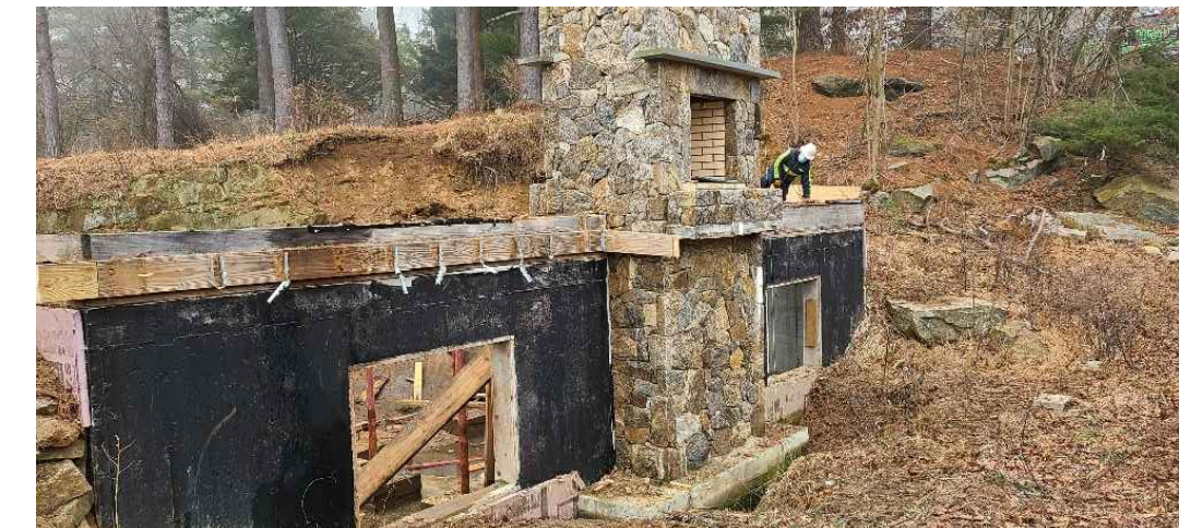
26 VIEW TO LAKESIDE (FRONT) OF CABIN DURING DEMOLITION. FIREPLACE IS DOUBLE SIDED WITH IN DOOR AND OUT DOOR FIRE PLACES. A NEW DECK WILL REPLACE THE DAMAGED DECK RECENTLY DEMOLISHED AND REMOVED FROM THE PROPERTY
