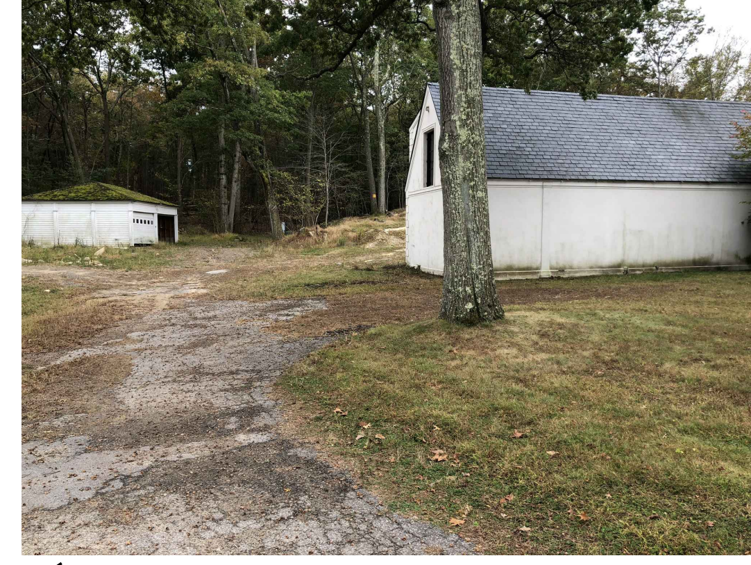
11 VIEW SOUTH TO EXISTING GARAGE AT LEFT OF PHOTO AT SOUTH CENTRAL PROPERTY. GARAGE TO BE RENOVATED.
