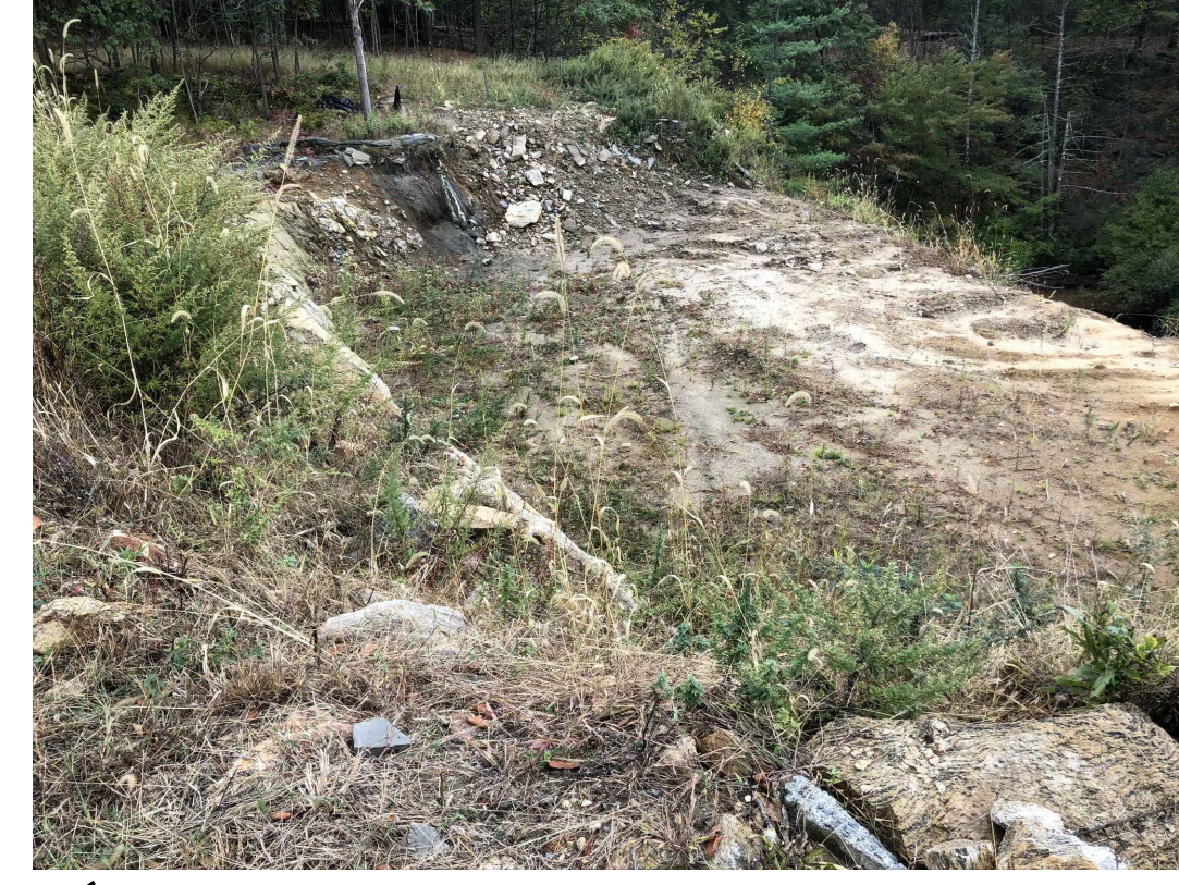
10 VIEW OF EXCAVATED FORMER PATIO AREA WHICH OVERLOOKS LAKE. NEW PATIO AND GAZEBO OVERLOOK ARE PROPOSED.
