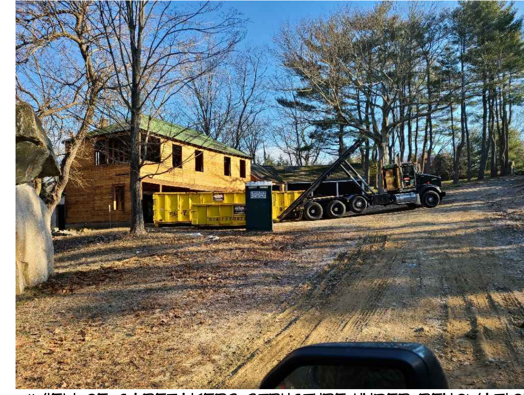
18 VIEW OF CARETAKERS STRUCTURE UNDER RENOVATIONS. NOTE THE ADJACENT AREAS HAVE NOW BEEN CLEANED OF PREVIOUSLY STORED CONSTRUCTION MATERIALS AND CONSTRUCTION DEBRIS
