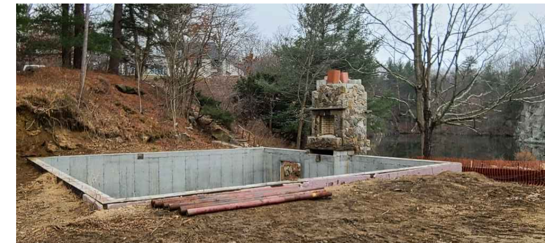
25 VIEW TO CABIN FOUNDATION TOTALLY REMOVED OF DAMAGED STRUCTURE. NOTE THAT ADJACENT SITE AREAS HAVE NOW BEEN CLEARED OF SCATTERED DEBRIS AND WASTE.
