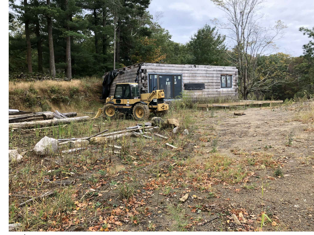
16 VIEW TO DAMAGED LAKESIDE CABIN. REQUIRES RECONSTRUCTION. EXISTING DILAPIDATED STRUCTURE HAS BEEN REMOVED
