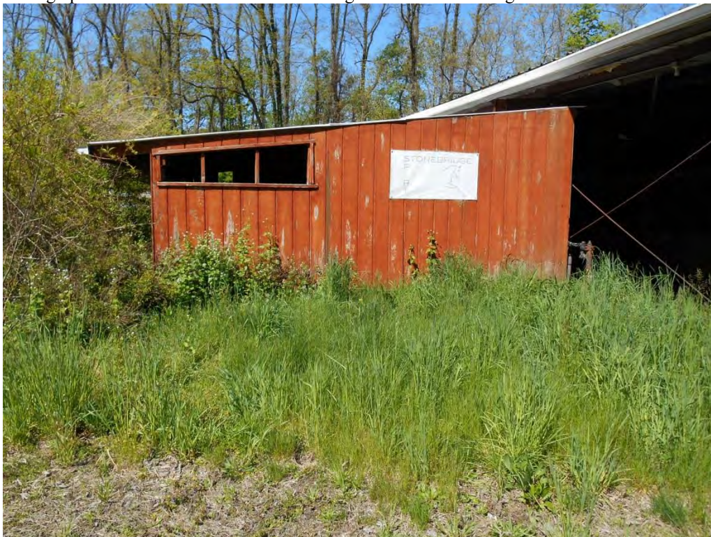
Photograph 6. Detail of the shed addition to the indoor riding arena that is proposed to be demolished. View looking southwest.
