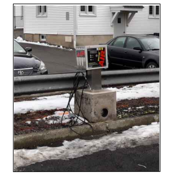
PHOTO 4 : EXISTING AIR PUMP
