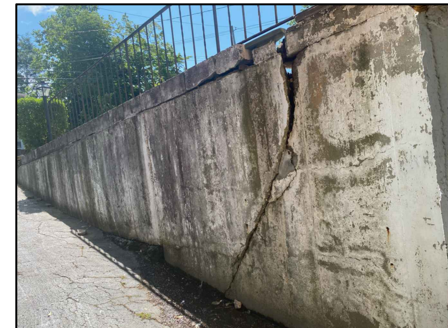
EXISTING FAILED CMU RETAINING WALL AND GUARD RAIL
