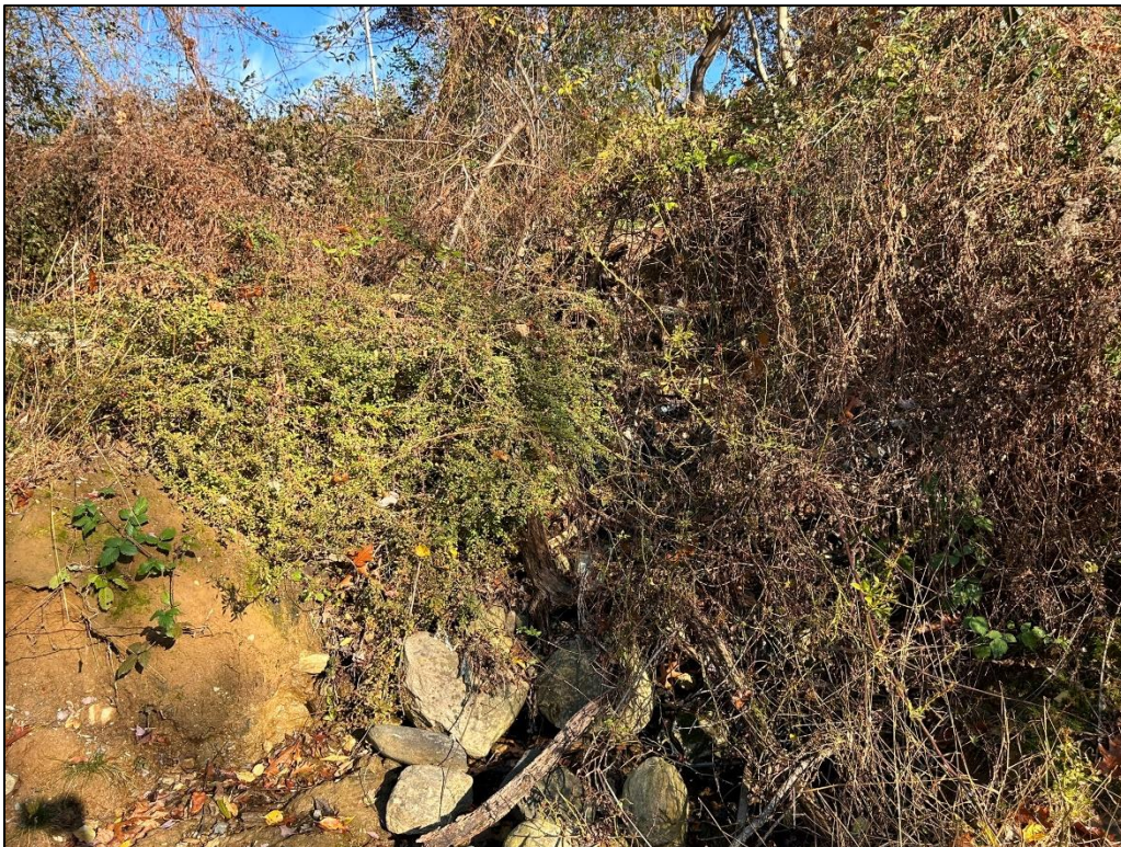
Photo 16. Looking east from the top of the Y-shaped drainageway where the roadway drainage leaves a pipe and cascades onto the site along a rocky spillway.
