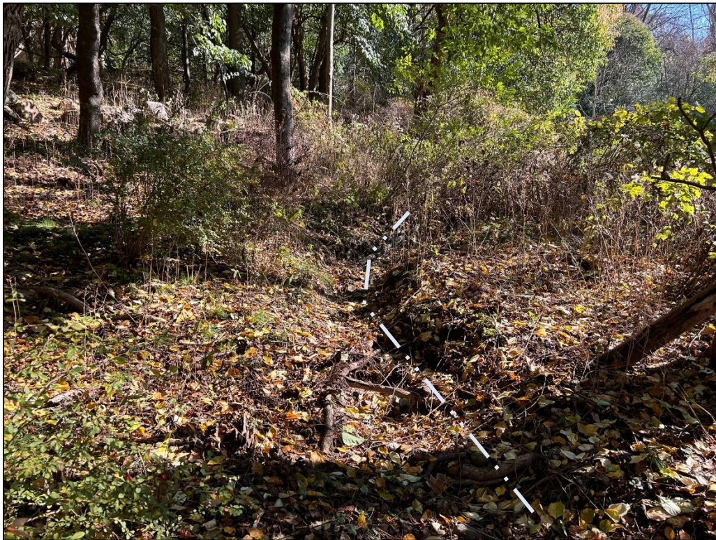
Photo 10. Looking east at the bottom of the "linear drainageway" which conveys stormwater from Byram Ridge Road into the wetlands. Shown by dashed line.
