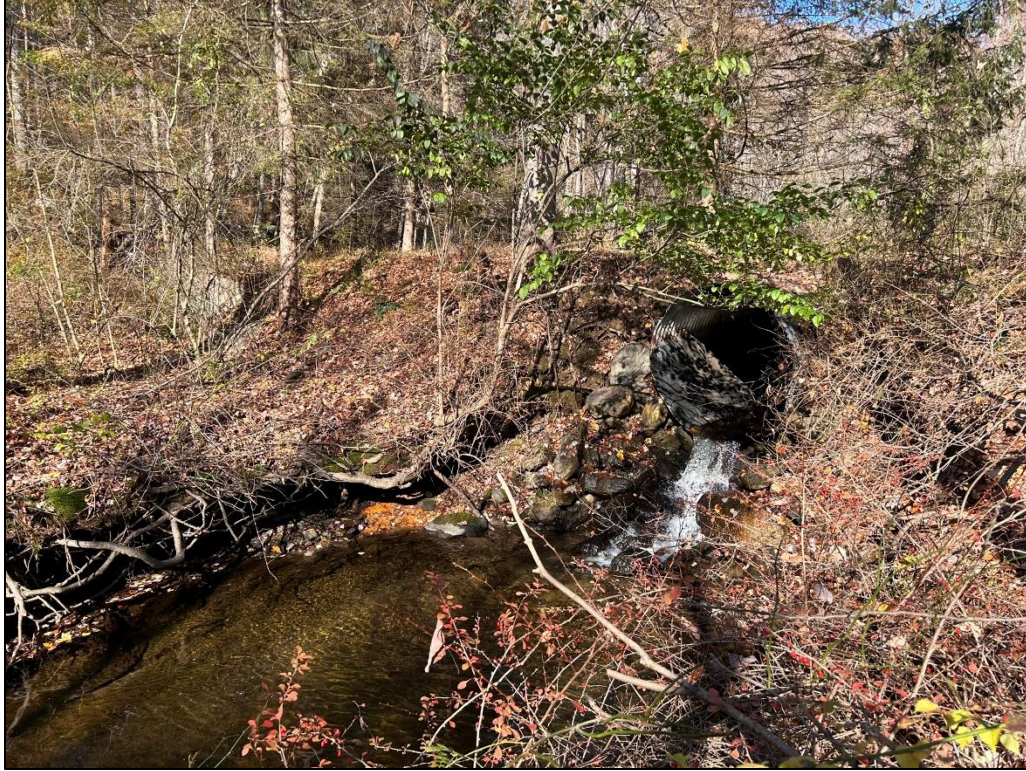
Photo 1. Looking north at the large stream culvert which feeds the watercourse/stream on the northwest portion of the site.
