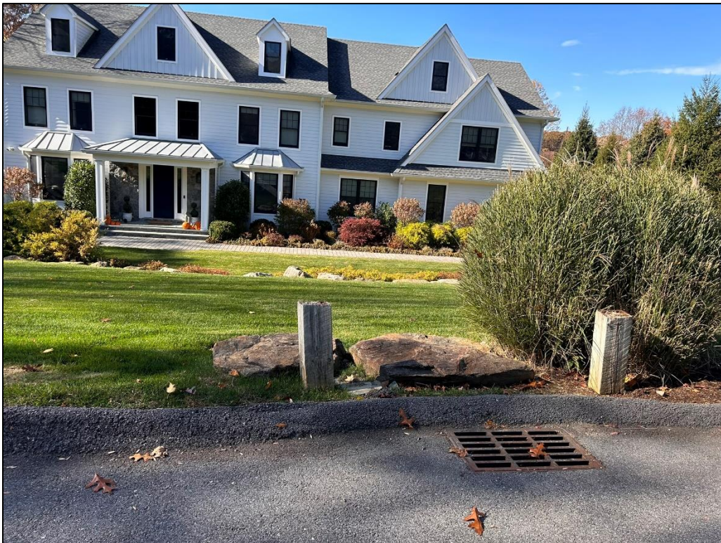
Photo 14. Looking at the drain at 85 Byram Ridge Road which conveys water underground and dumps it on the site.
