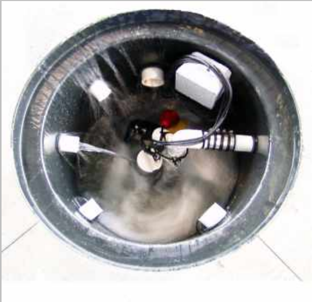
PRIMARY COLLECTION SUMP
