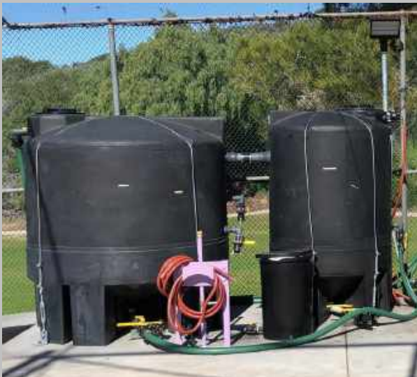
CLARIFIER & WATER STORAGE
